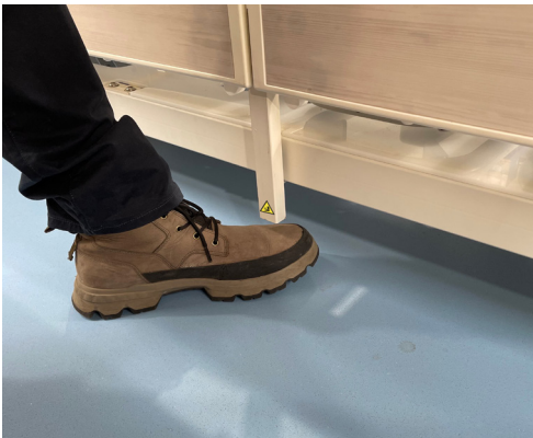
The gap between the underside of the side rail post and the floor.
